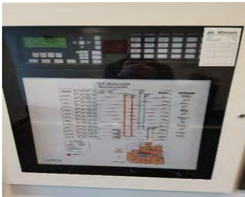
Item 58 - Fire Alarm Panel
