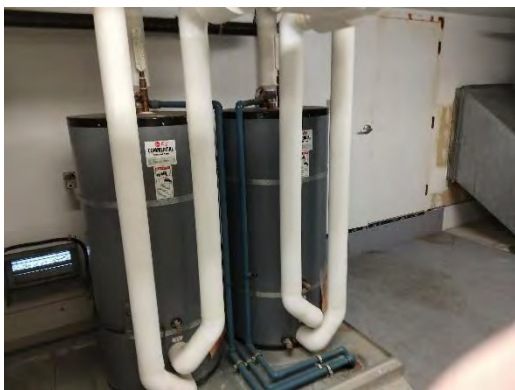
Item 42 - Domestic Hot Water Equipment
