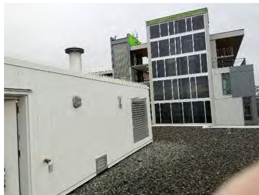
Item 9 - Mechanical Penthouse
