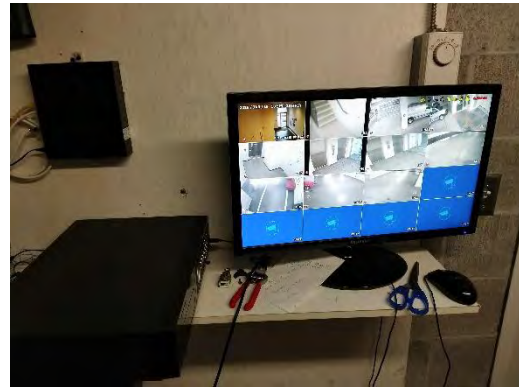
Item 59 - Video Surveillance System
