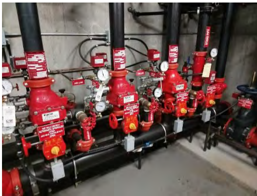
Item 55 - Fire Pumps
