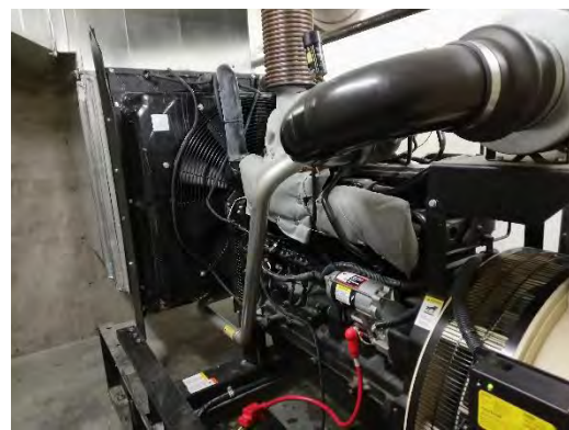
Item 63 - Emergency Generator
