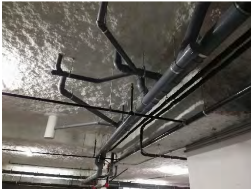
Item 45 - Waste Water Piping
